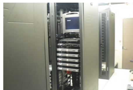
SDS's new Data Centre
